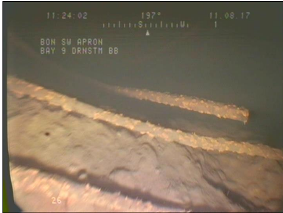
Figure 10 Additional imagery of erosion on downstream side of baffle blocks at SB 9.
