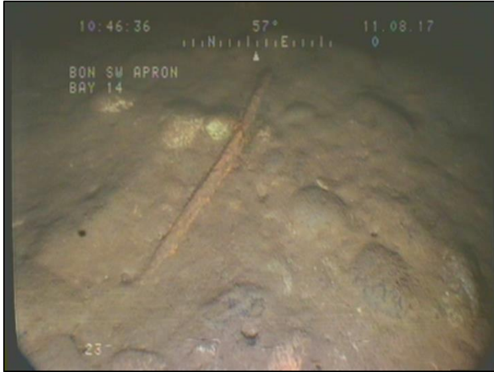
Figure 8 Exposed rebar in SB 14.
