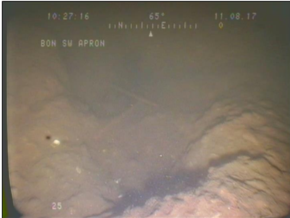
Figure 13 Typical erosion and exposed rebar found at the downstream corners of all baffles in the first row.
