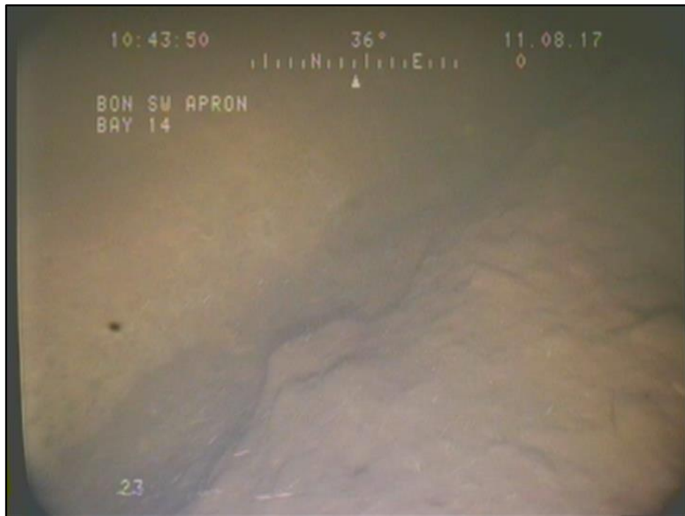
Figure 7 Erosion found in SB 14 between the 2012 concrete repair and the 13/14 dividing pier.
