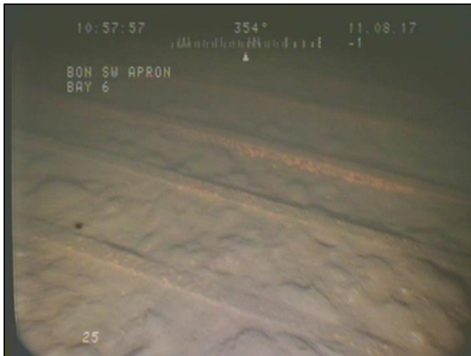
Figure 11 Erosion and rebar found upstream of baffles at SB 6.
